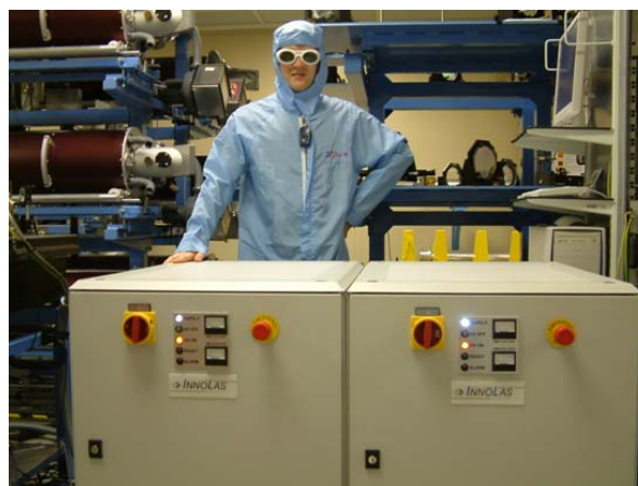
Figure 2. Two of the Innolas 9mm amplifier power supplies installed in Vulcan.
